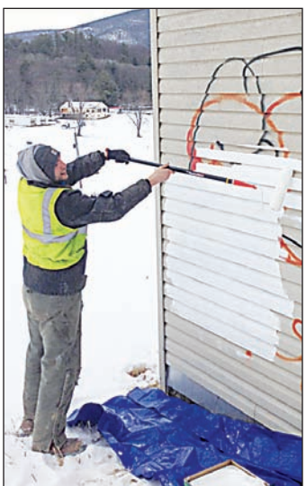
A worker covers the graffiti on a building of the Spring Glen Resort.
