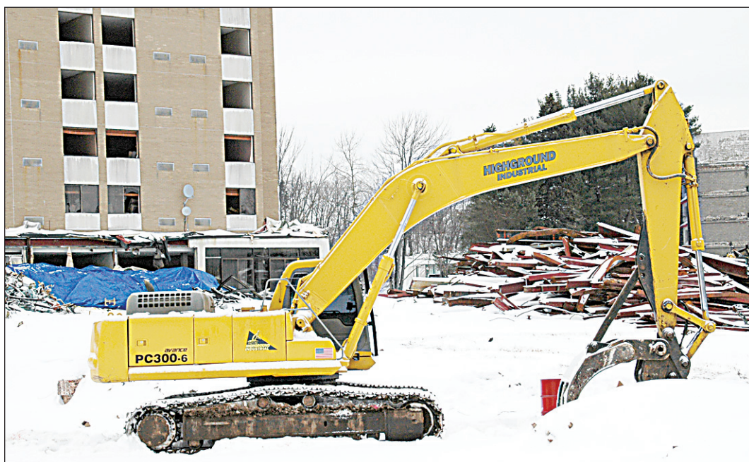
Demolition work quietly proceeds at the former Kutsher's Country Club near Monticello this week. Meanwhile, a new documentary about the famous, long-lasting resort is debuting this month and next.
